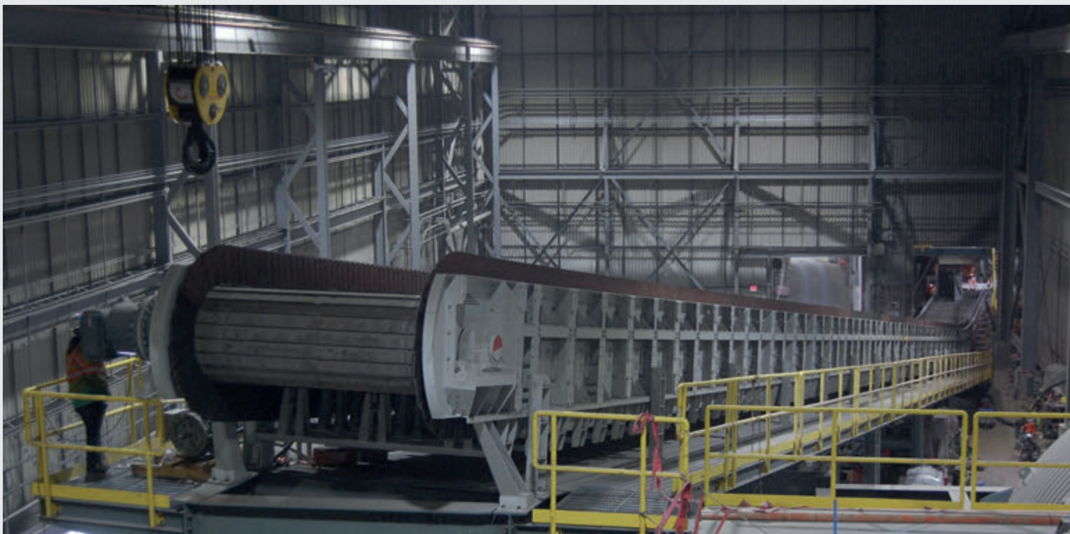
A huge heavy-duty Superbelt conveyor handling steel scrap to feed a pre-heating system in an integrated steel mill.
